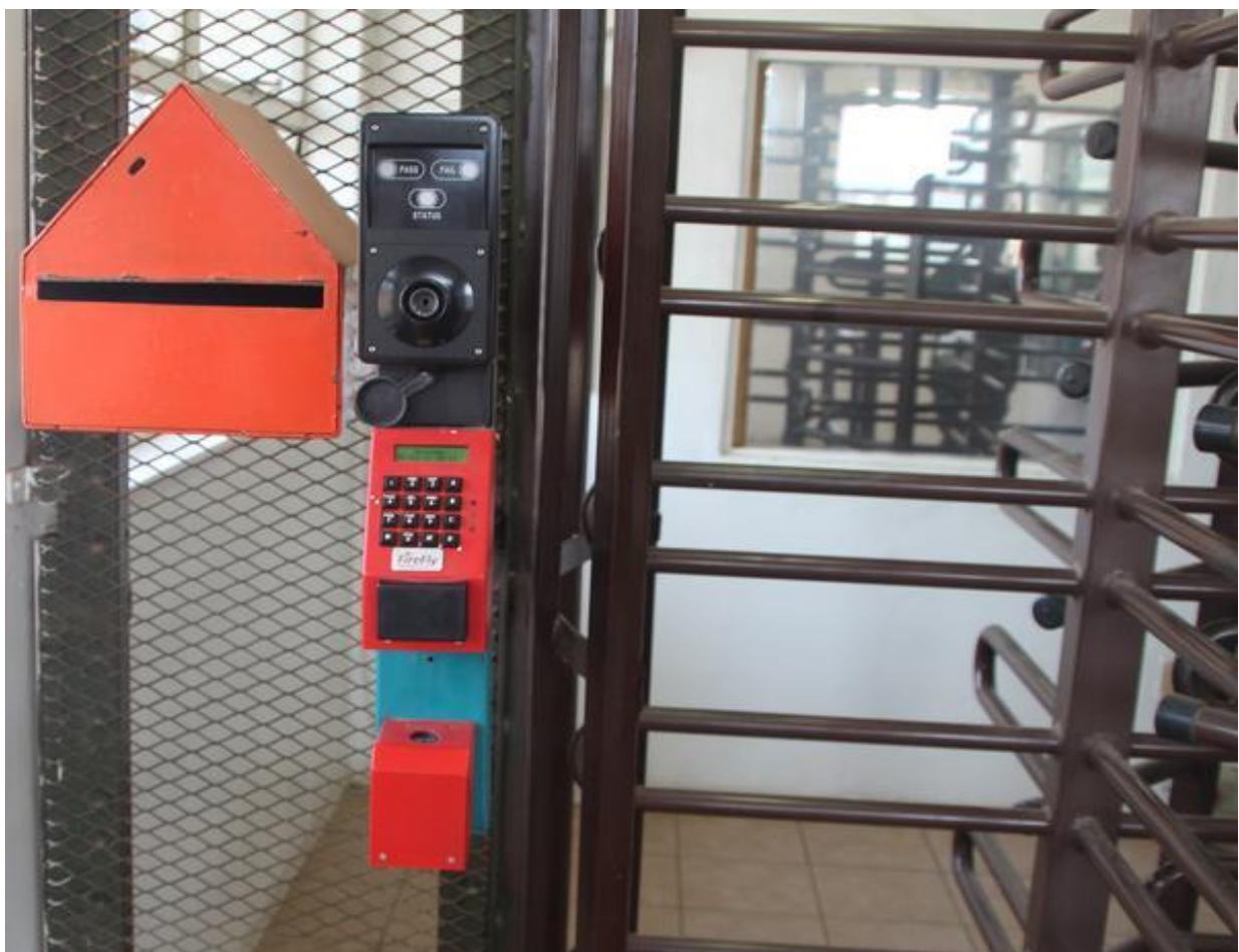
Fig 13 showing the integrated system with the turnstile to the car park
