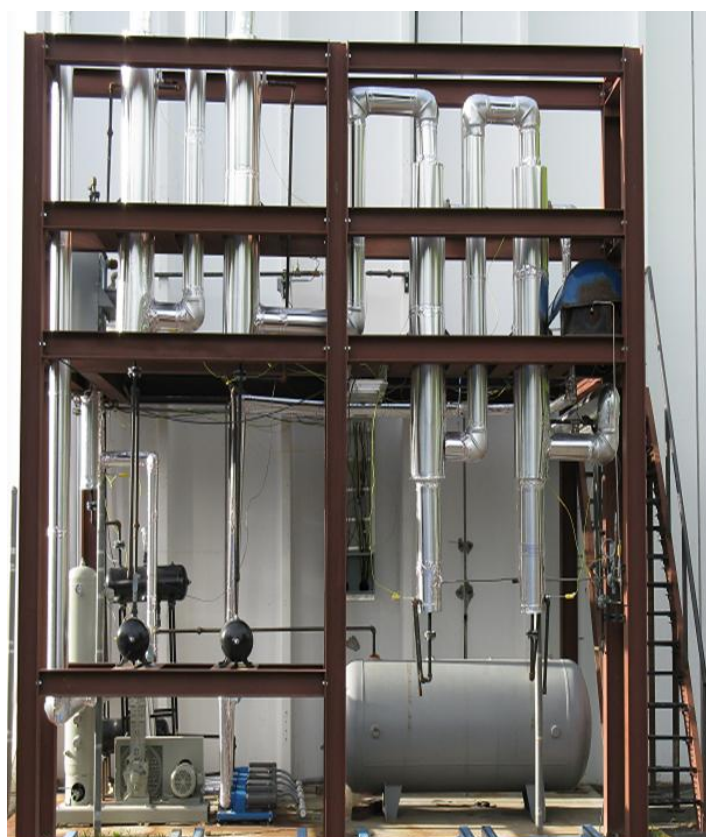
Figure 4 – distillation unit, induced draft fan and storage tank
