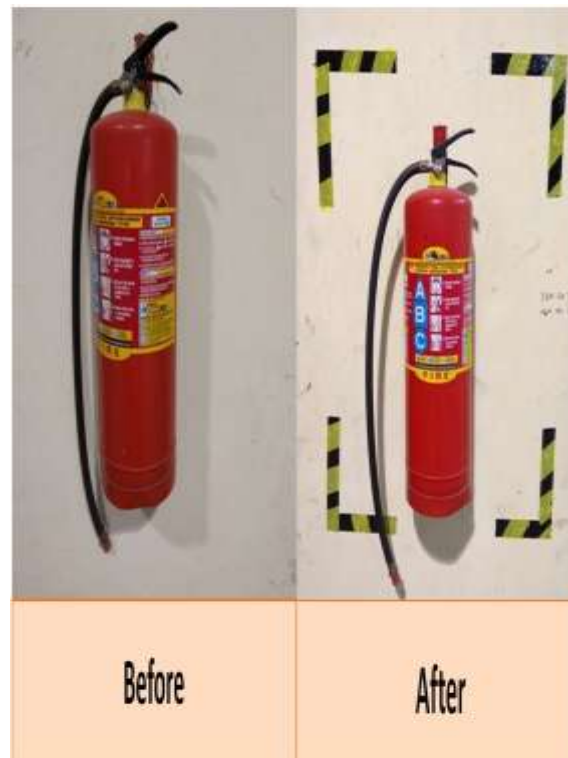
FIG 22:Photograph before and after(Location for fire Extinguisher)
