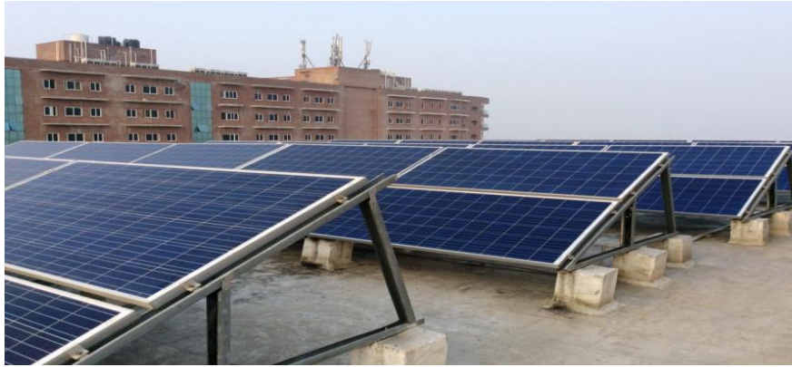
Fig. 1: View of 1 MWp rooftop grid-connected solar PV system.
