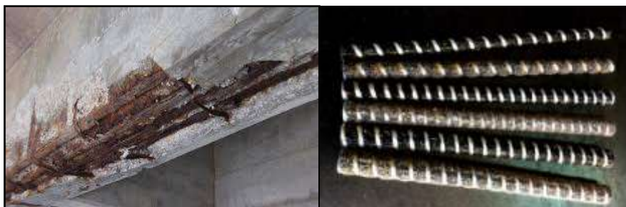
Fig.1 Corrosion in reinforcement Fig.2 Basalt Fiber Reinforced Polymer bars
