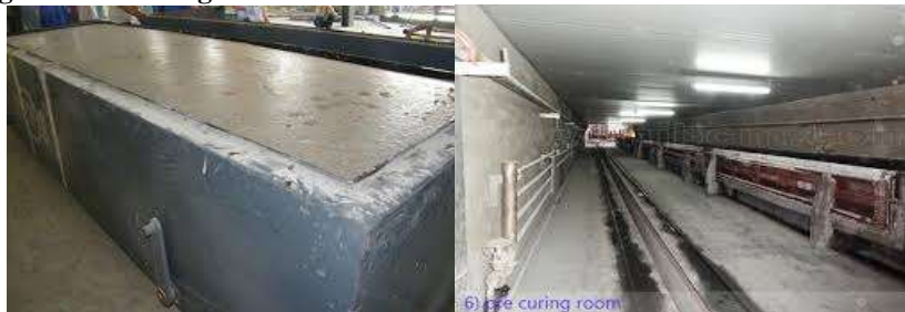
AAC BLOCK PRODUCTION LINE
