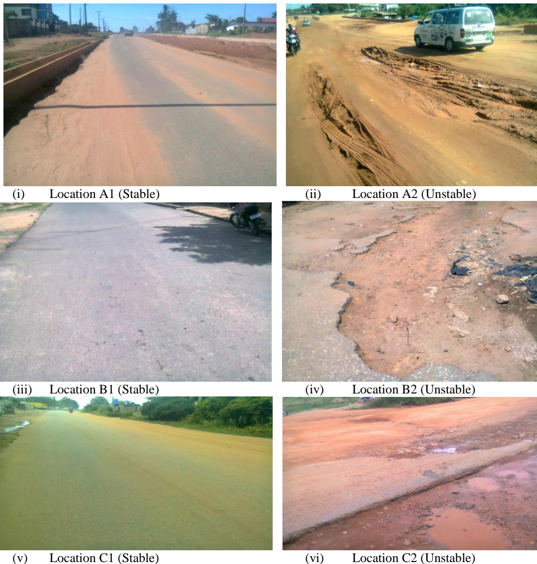
Figure 3: Stable and failed road sections adjacent to sampling locations in Owo [i] and [ii]; Iworo [iii] and [iv]; and Ikare-Akoko [v] and [vi].
