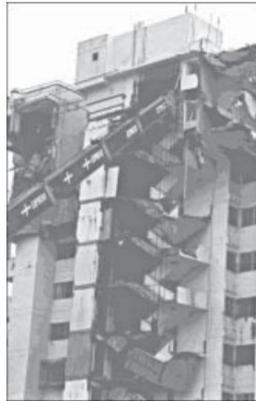
Fig 2. Failure of signboard in Bhuj earthquake, 2001
