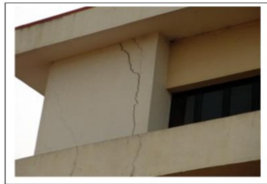
Plate 2b: Severe cracks noticed on the structure
