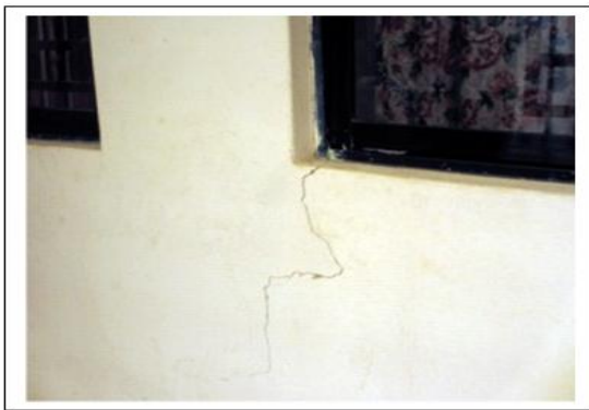
Plate 2a: Mild crack noticed on the structure
