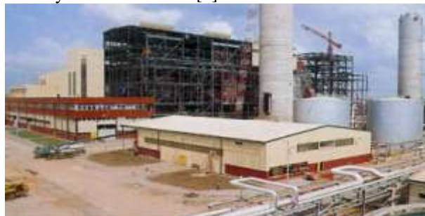
Figure 1: Nigeria Power Station
