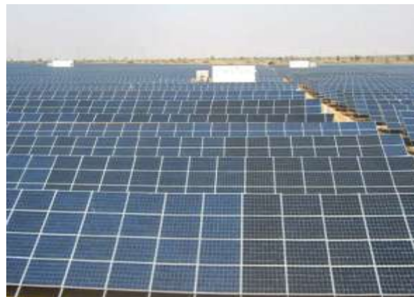
Fig.3: Dhirubhai Ambani Solar Park, Rajasthan
