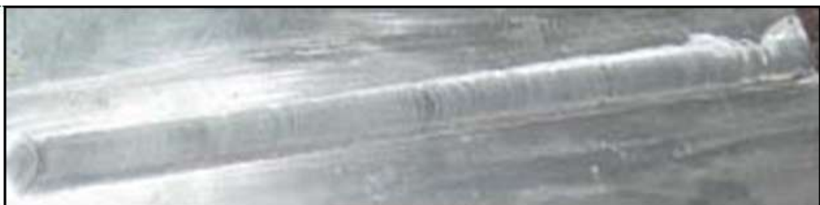
Figure 4.1(a): Close-up view of a weld.
